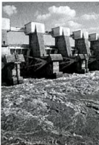
Gates of the Auxiliary Control Structure
