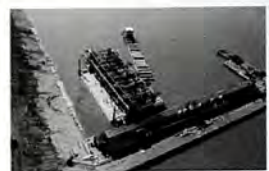
Reinforcing banks with revetments below the water line and concrete pavement above [U.S. Army Corps of Engineers]
